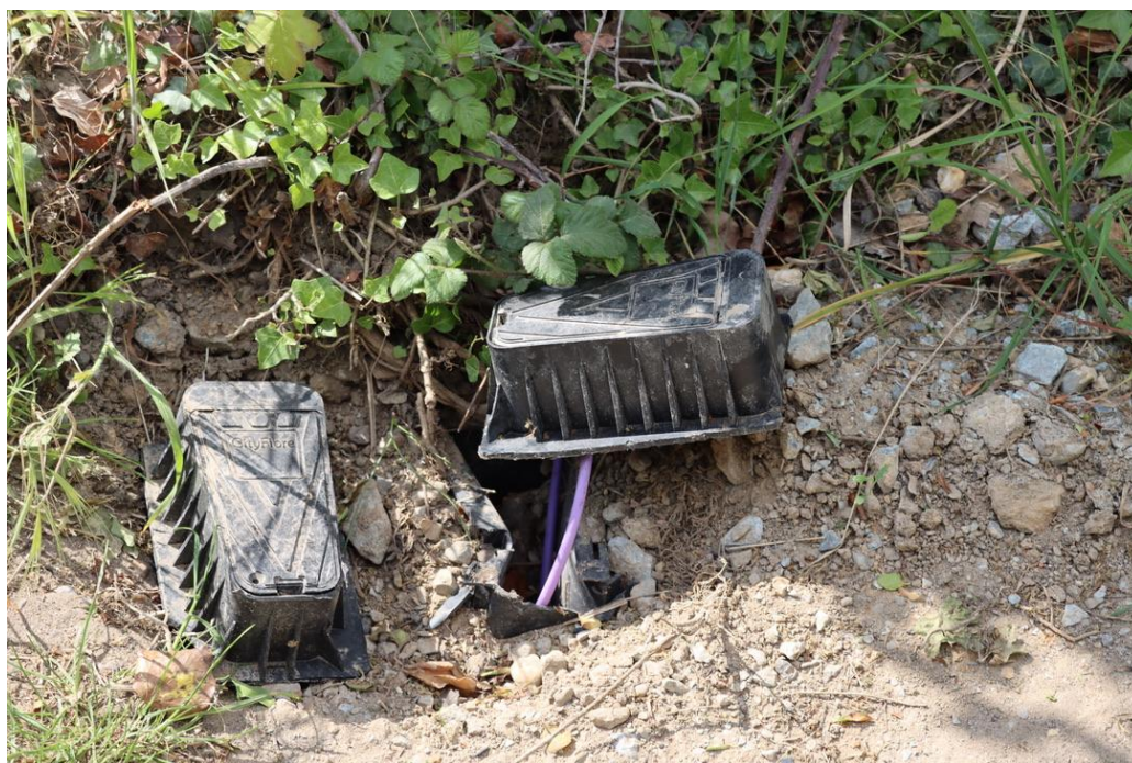
The overall excellence of City Fibre work may be judged by the image above: a cable installation in Thorpe Lane which lay exposed to the elements for at least a month.
